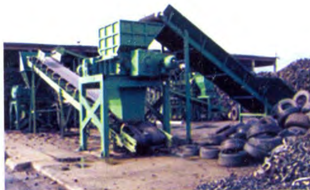
A Tyre Shredding System
