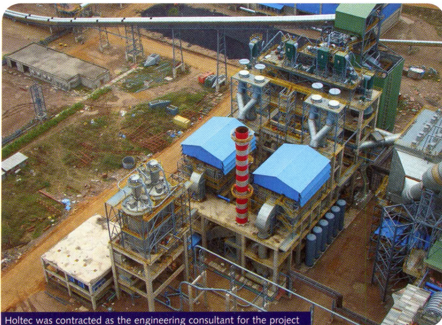
Holtec was contracted as the engineering consultant for the project
